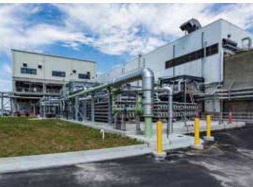
The new Cooling Facility for the HRSD's Atlantic Treatment Plant THP Improvements project will support the new Cambi THP.
