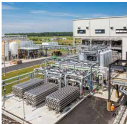
The Cooling Facility and Cambi THP prepare for commissioning in Virginia Beach.
